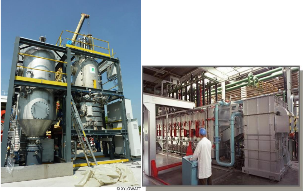
Figure 4 - Biomass gasifier and combustion test cell for BioVive Project
